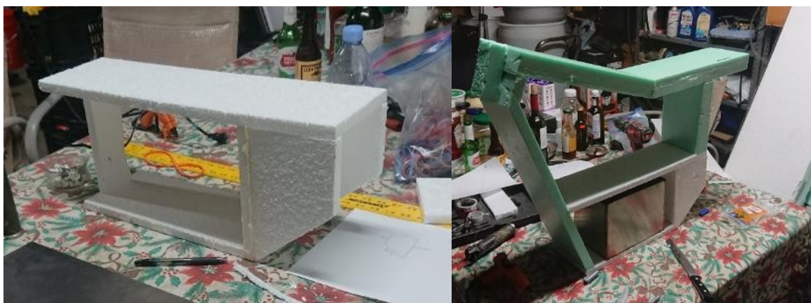
Fig. 5.3.1 The beginning of the construction of the EPS and XPS foam frame
